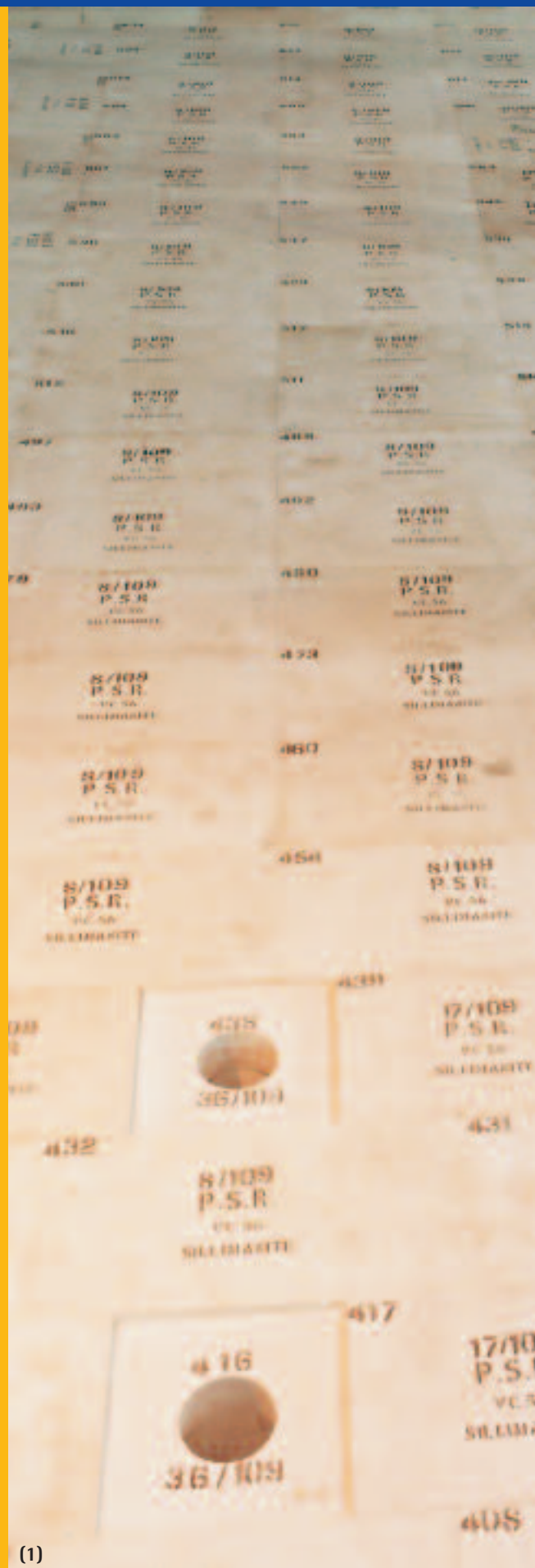
PSR Furnace bottom blocks are used in all sectors of the glass industry. Photograph (1) illustrates construction of a container furnace bottom prior to installation of paving tiles.
