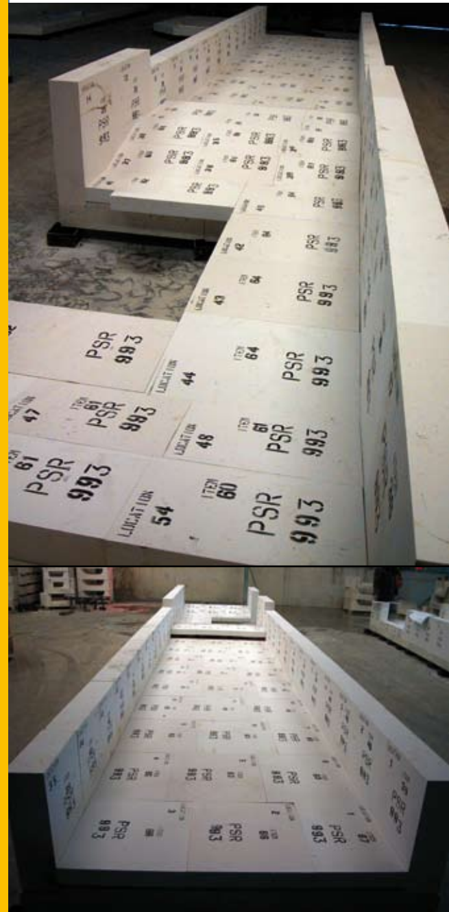
Pre-assembly of distributor glass contact blocks in PSR-993
